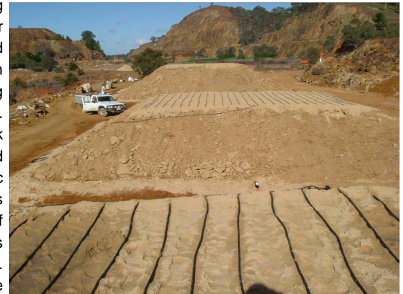
Alkalinity producing cover field demonstration at a mine site in South Australia.
